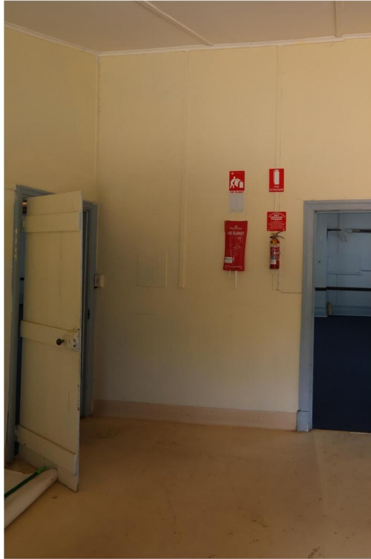
FIGURE 8: IT COULD BE PRUDENT TO ESTABLISH THE EXTENT OF ASBESTOS IN THE BUILDING.
