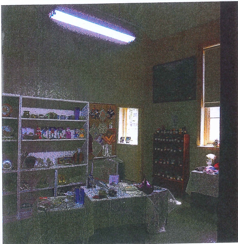
Interior: The c.1976 partition wall towards the south end of the 1894 school room showing the doorway through to the Museum section. Window 3 (right).
