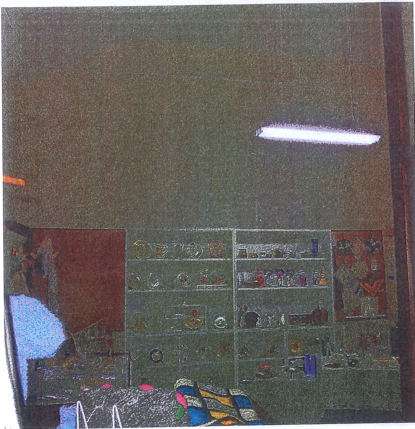
Interior: The c.1976 partition wall towards the south end of the 1894 school room.
