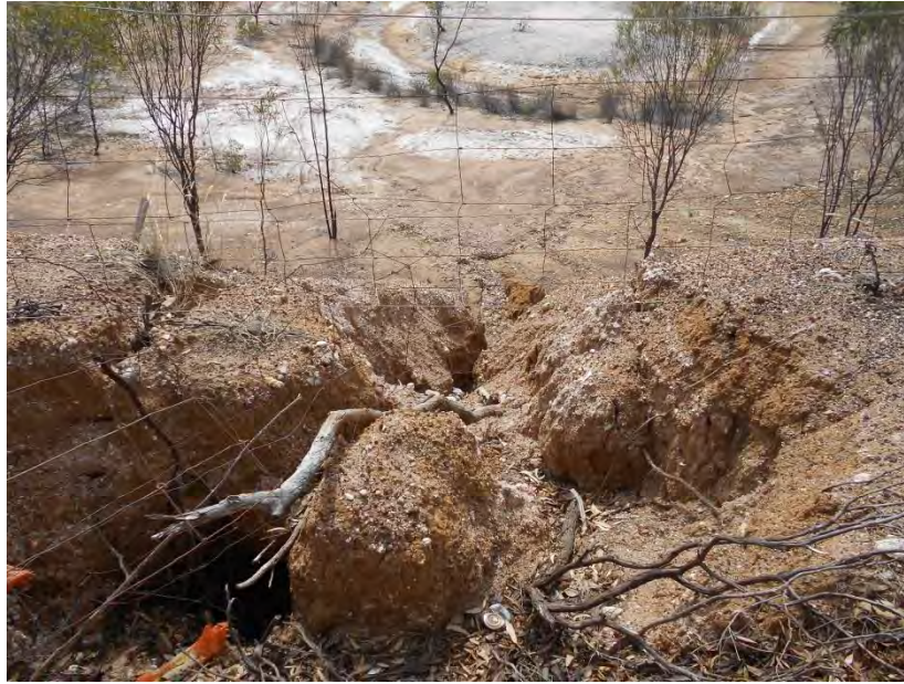
Plate 1: Erosion (and fencing) on banks of Archibald Park
