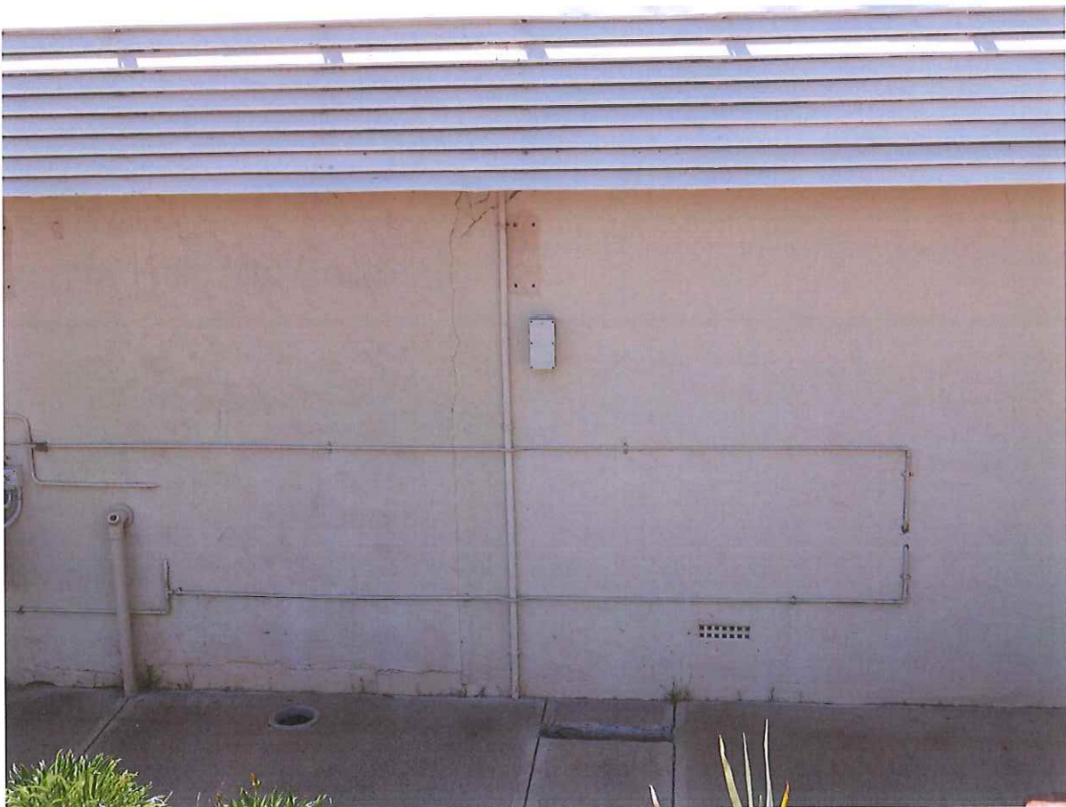
Figure 2; Photo of minor cracking in western wall of existing building.
