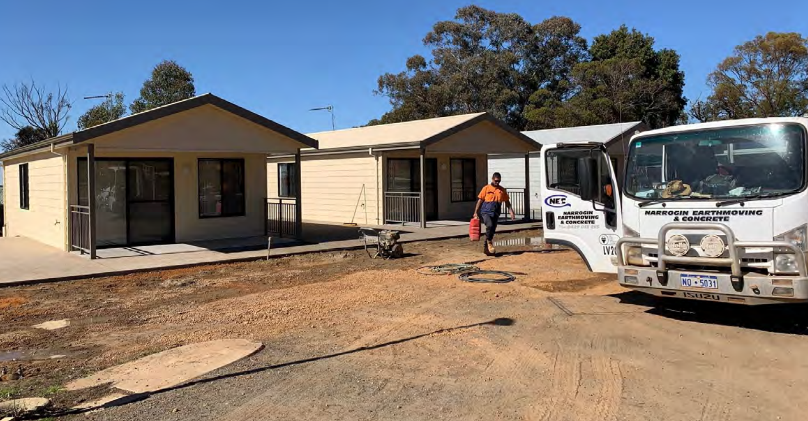
The construction of three Accessible accommodation units at the Narrogin Caravan Park
