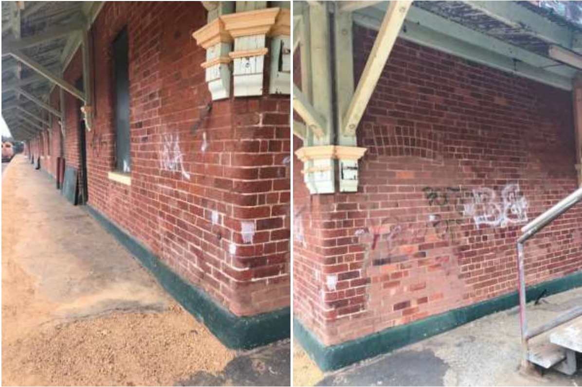
Photos 13,14 Narrogin Railway Station Details of the walls at the north end and to part of the east wall, showing interventions and graffiti on the face brick work.
