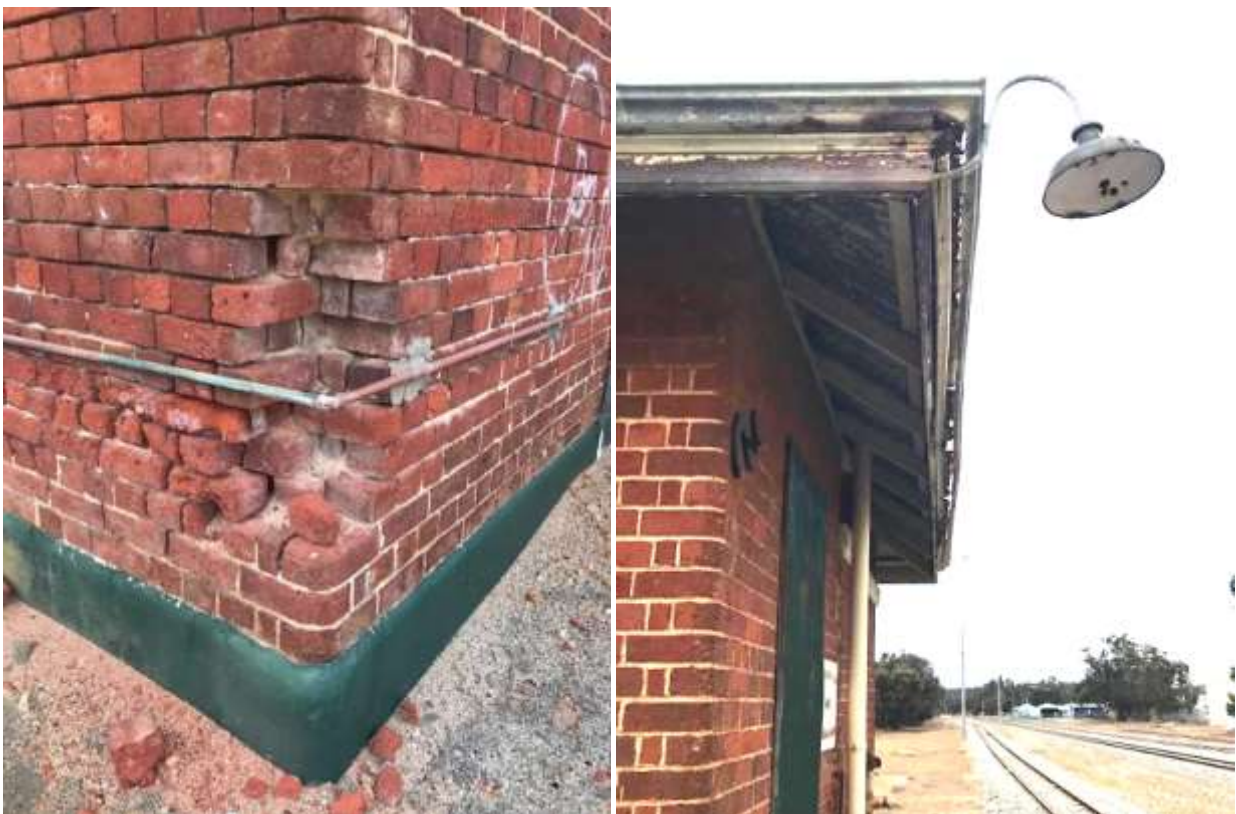
Photos 63, 64 Narrogin Railway Station Ablution building showing the southwest corner damage and erosion to the bricks and mortar in that location; and the roof trim weathered, and gutters rusting.
