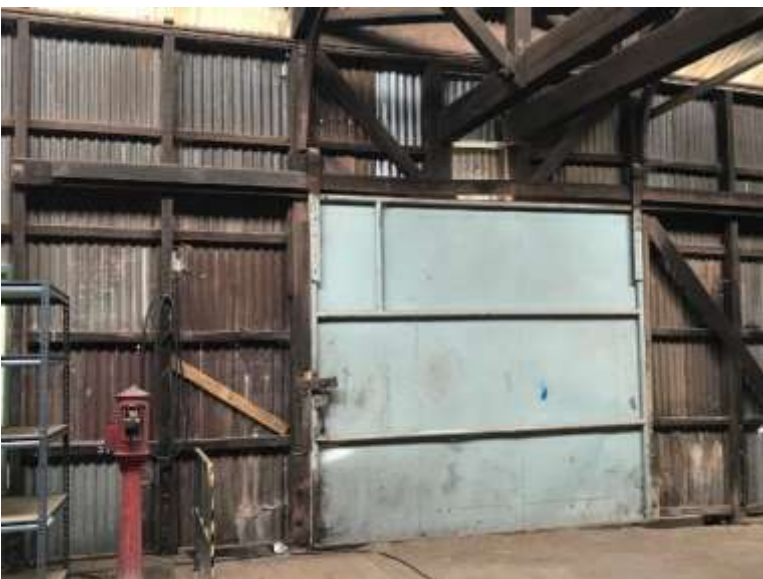
Photos 115-117 Goods Shed . Interior. Views of the roof structure; typical sliding door at loading bay.
