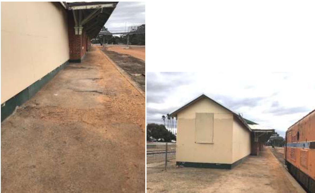
Photos 23, 24 Narrogin Railway Station View looking north along the east platform showing platform damage. The south end framed and clad addition was not accessible.
