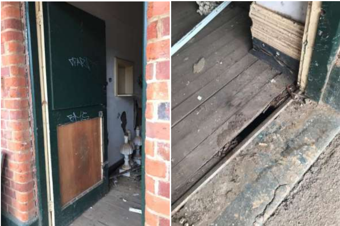
Photos 17,18 Narrogin Railway Station Entry into the second room along the east of the station, showing damaged door and threshold.
